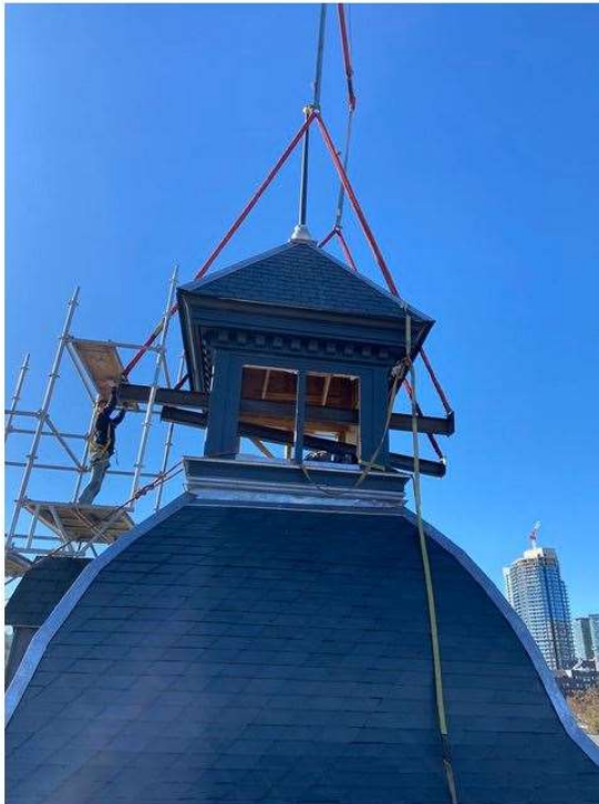
The new lantern being lowered into place at the Winchester Hotel in Cabbagetown.
